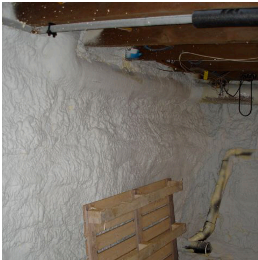
Water-blown, bio-based, closed-cell spray foam on basement walls improves indoor air quality by reducing dampness, while enhancing energy performance.
